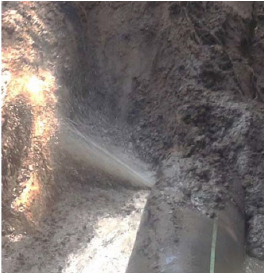
Figure 1. There is more than one way to repair leaks in large pipelines without shutting down operations, losing pressure, or risking the need to issue a boil-water advisory – including temporary clamps, line stop and bypass strategies, and permanent encapsulation.
