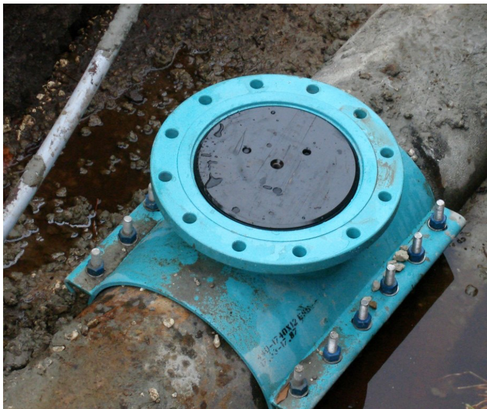
Figure 3. Once the pipe repair is completed and the bypass line removed, all that will be buried underground is the line-stop fitting with a plug (shown in black) that gets topped and protected by a blind flange.
