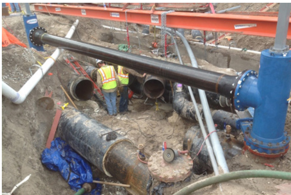
Figure 1. Bypassing the shortest length of pipeline needed to repair the original problem isolated between the line-stop fixtures minimizes the number of service connections that need to be disrupted for the duration of the repair effort.
