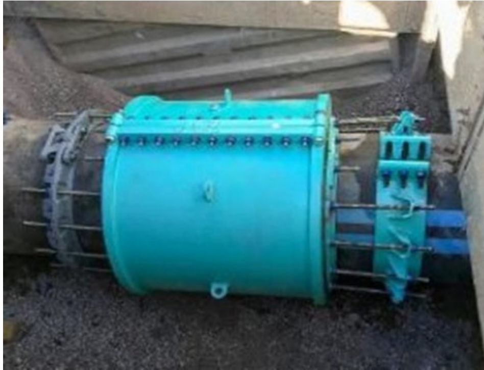
Figure 2. Full encapsulation of the original problem and the temporary repair clamp can provide peace of mind for the remainder of a pipeline's life expectancy.
